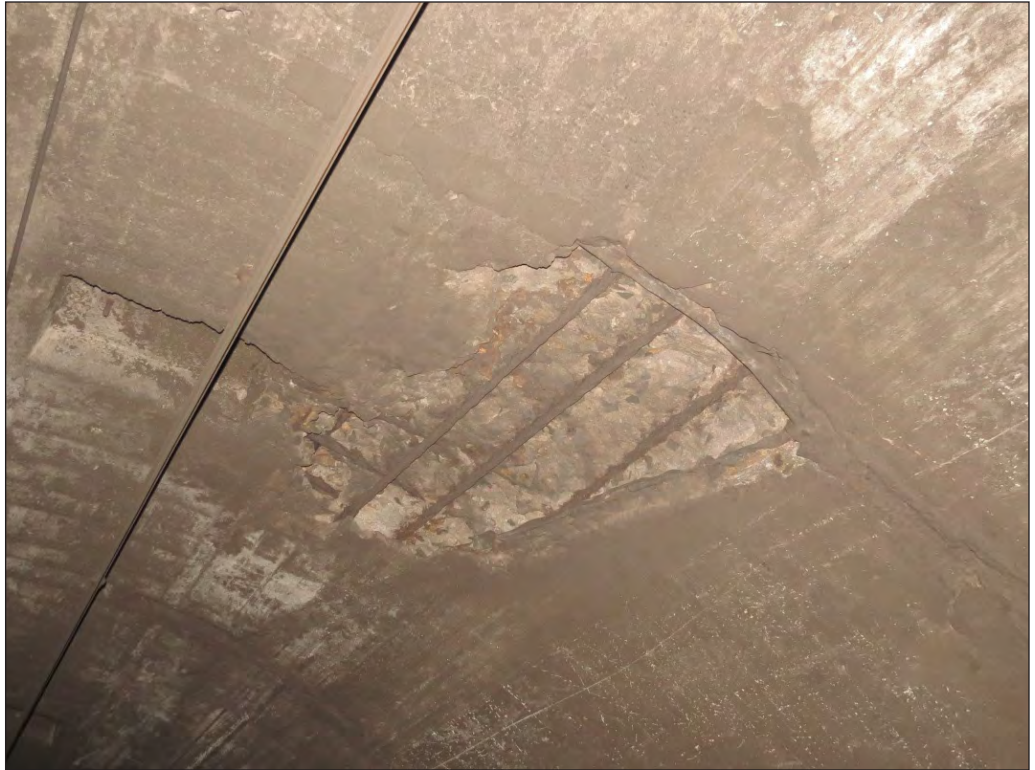
North River Tunnel damage, concrete lining
