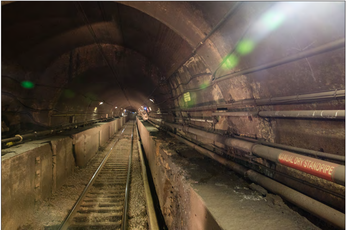
North River Tunnel showing damage including the bench walls and concrete lining
