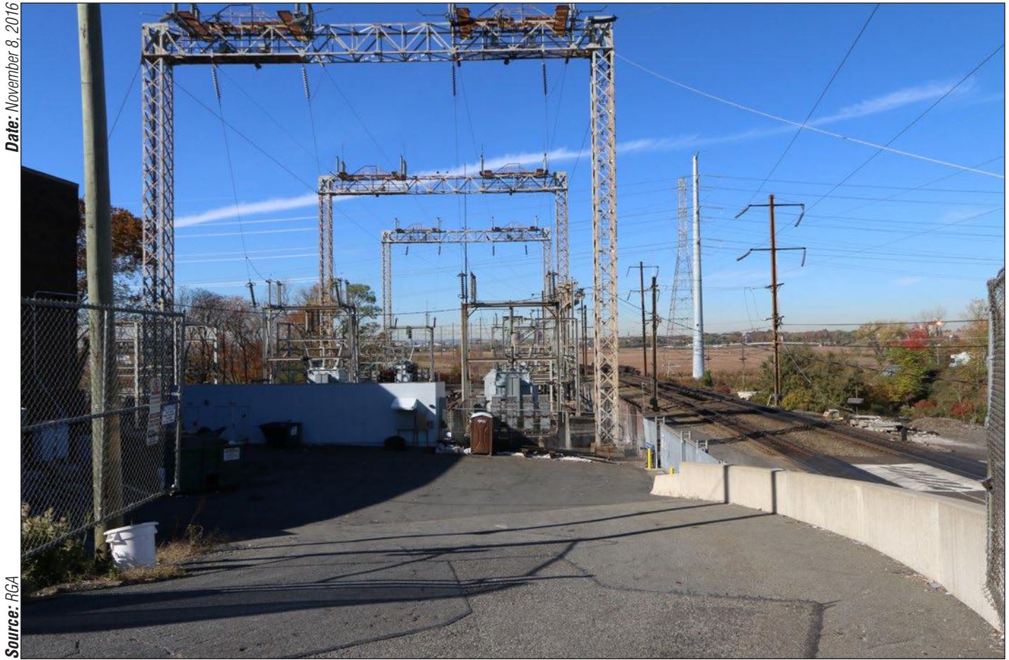
View west of Amtrak's Substation 42 at left and the NEC / PRR Historic District at right from Tonnelle Avenue in the Township of North Bergen. The New Jersey Midland Railway/New York, Susquehanna and Western Railroad (NJMR/NYSWRR) Historic District runs north/south directly behind the substation.
